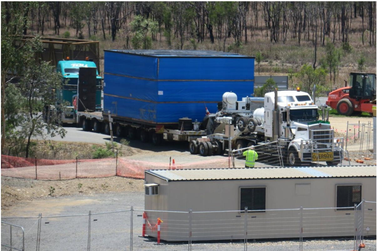
Oversize equipment for the construction of the AUS $75 million Tableland Green Energy Power Plant.
