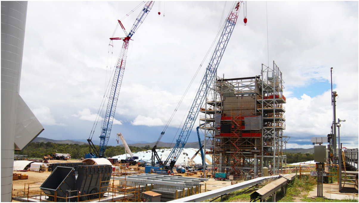
Full steam ahead - Construction of MSF Sugar's Tableland Green Energy Power Plant project is on track for a mid-2018 completion. (Picture from MSF Sugar)
