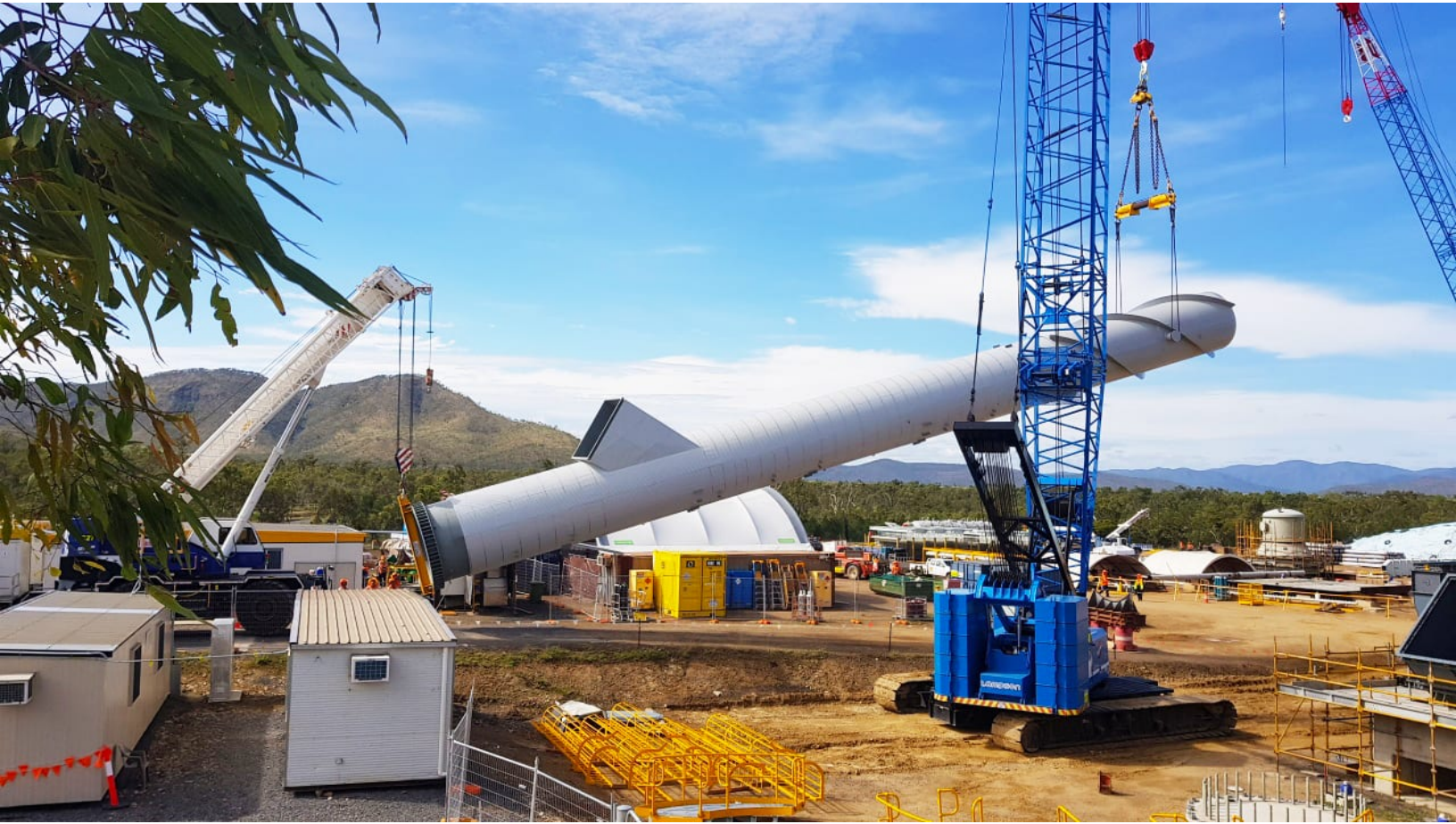
A 38.35m chimney stack is erected at MSF Sugar's Tableland Green Energy Power Plant. (Picture from MSF Sugar)
